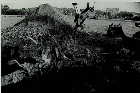
With the aid of a heavy crane, a German anti-aircraft gun is excavated from Meinerswijk polder near Arnhem on 30 August 1996. The barrel, which the retreating Germans had blown off, is lying alongside and is not visible in the photo.
